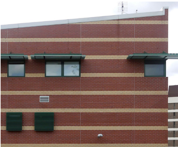
Fig. 5 Detail, Roma Street Fire and Ambulance Station, Brisbane, 2007, Project Services (Design Architect: Spence Jamieson). Photograph by Ashley Paine, 2014.
