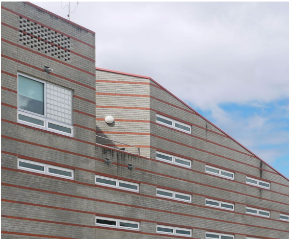
Fig. 4 Detail, Block B, SQIT, Toowoomba, 2002-6, Project Services (Design Architect: Donald Watson). Photograph by Ashley Paine, 2015.
